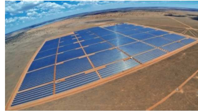
PV panels on the 50 MW Droogfontein solar PV project in the Northern Cape. Source: www.greenbusinessguide.co.za
